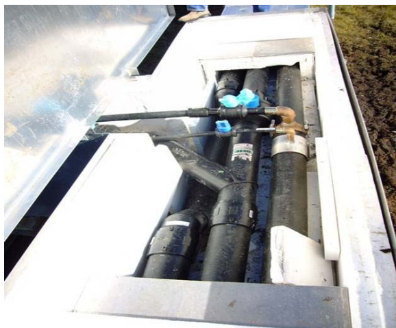
Figure 2: Photo of Existing Circulating Water and Vacuum Sewer Main within Utilidor
